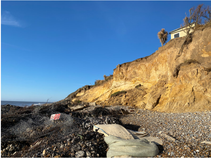
Appendix 3. Photos of current sea defence damage and erosion at Thorpeness (2021) (site shown is Pt 2 on the map)
